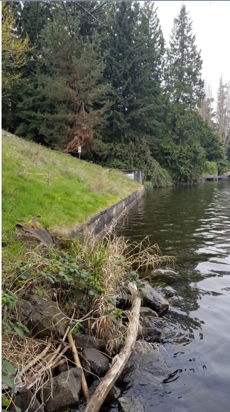
Photo 23. Mercer Island Boat Launch work area – Riprap placed into Lake Washington, presumed as support for failing bulkhead.
